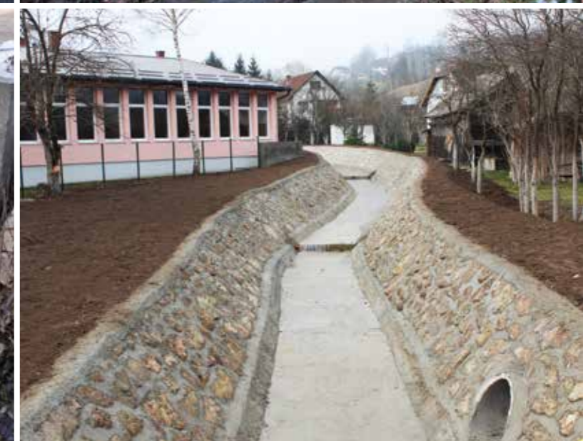
Olovo: Regulated streambed in Solun LC (protection of Hasan Kikić Elementary School)
