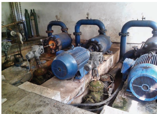
Hydromehanička oprema u pumpnoj stanici Krupić (HEIS, 2015)
